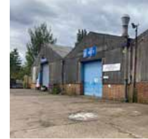
Mix of corrugated steel and brick work. Lack of windows enhances the industrial feel.
