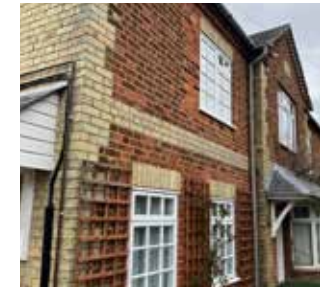
Red brick with sandy brick detailing including quoins and soldier course lintels.
